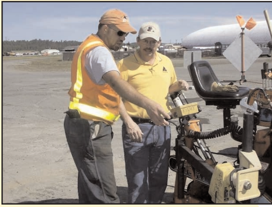
AI Field Engineer Mark Blow (right) shares the latest quality construction techniques with Elmendorf AFB personnel in Alaska.
